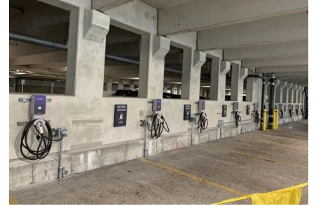
UMass Boston's EV Charging Infrastructure
