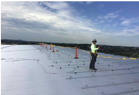
UMass Boston's Solar Photovoltaic System
