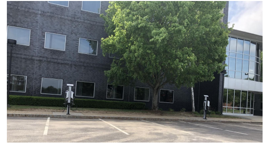
ENE's EV Charging Infrastructure
